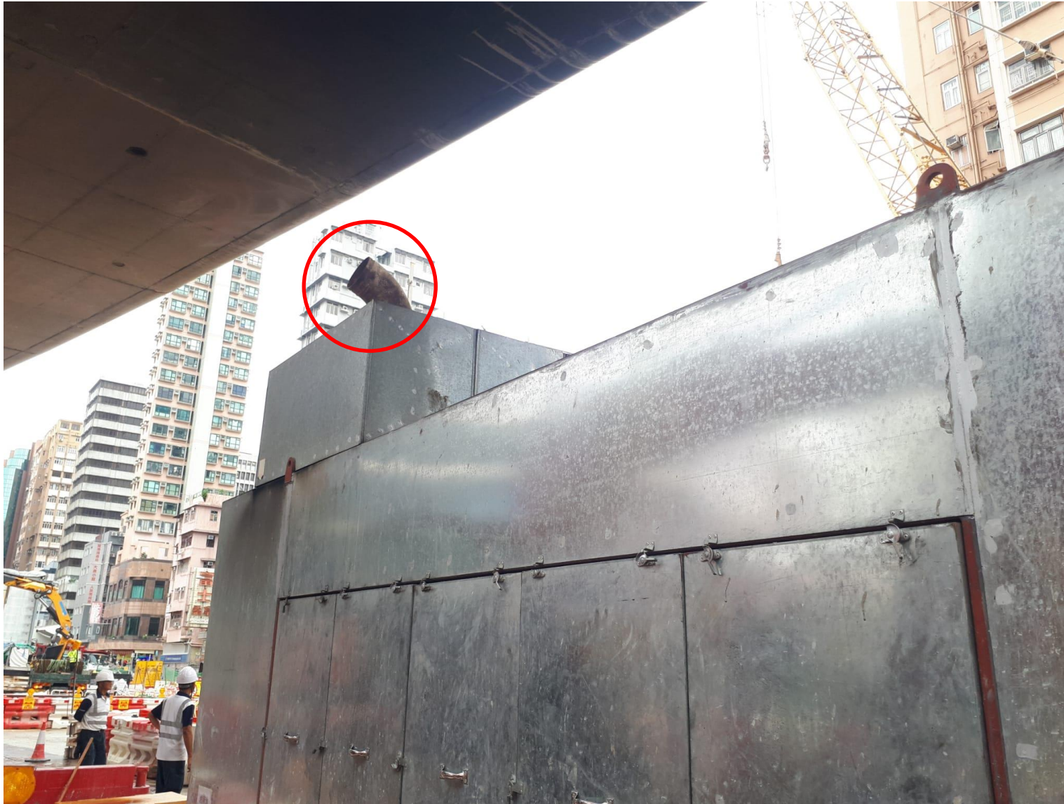
Remark 2: Mitigation measure of diverting the outlet exhaust
